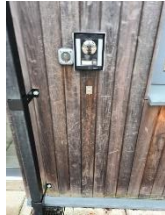
External intercom requires signage
